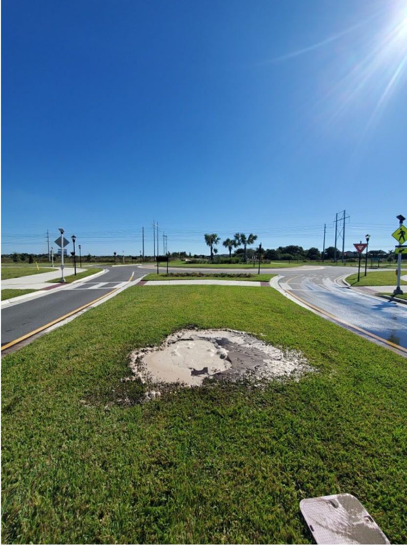
Mainline leak reported on October 18 th .
